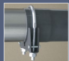
detail of the pipe connection of the heating tubes
