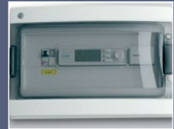
Siemens Climatix control box
