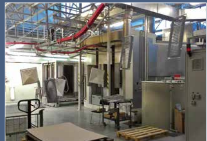
Powder Paint Shop
